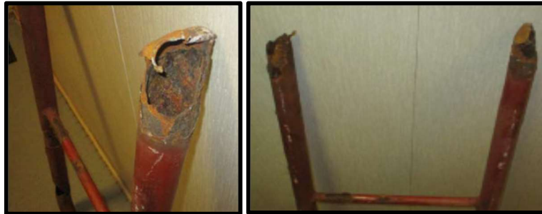
Picture 1: Closer examination of the railing revealed severe corrosion (metallurgy thinning) at the bottom joints
